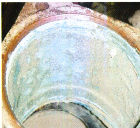
Fig. 14 Water box inner surface
