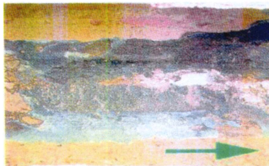
Fig. 7 CuNi tubestack through hole perforation, wall thinning, presence of black deposit, and oxide film
