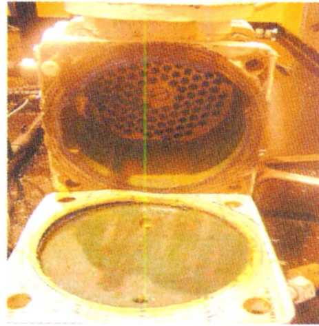
Fig. 10 Overview of HMS Sultan test rig water box inlet side assembly, after 8 weeks standing
