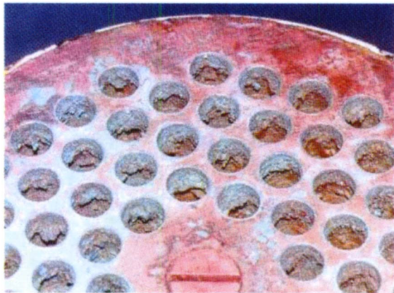
Fig. 4 Corrosion of the CuNi fixed end plate and deposits in the exposed tube ends
